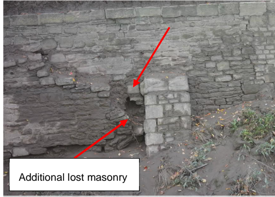
Figure 10.16: NCS28 Wall deformation 2022
