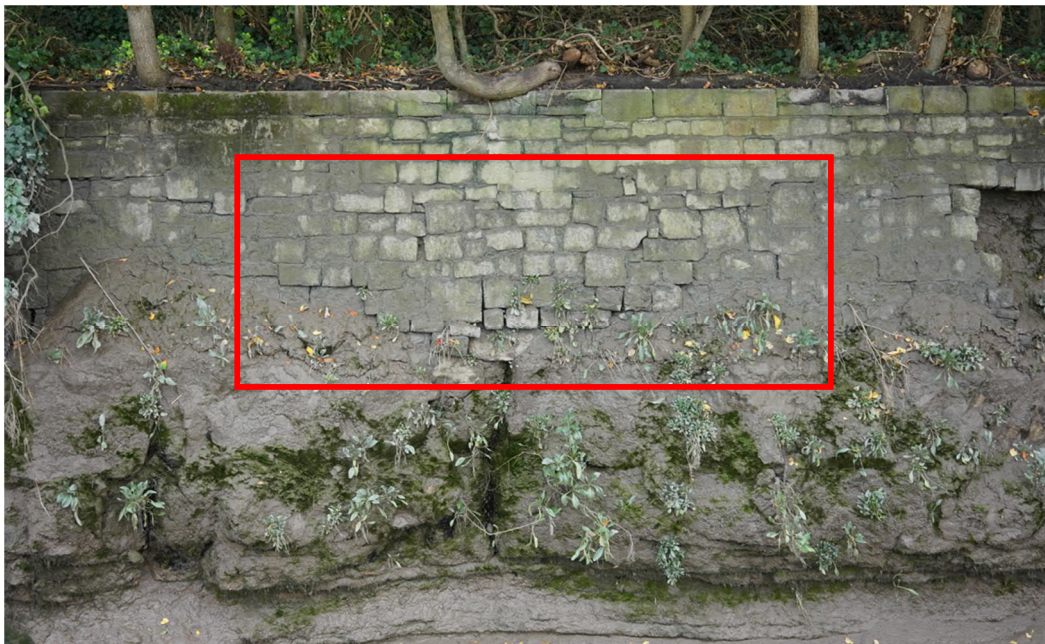
Figure 7.4: NCS13 Typical example of minor wall deformation
