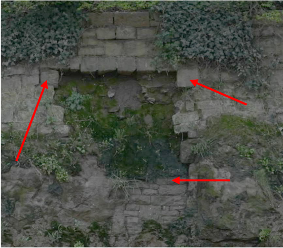
Figure 7.7: NCS13 Collapsed section 2019
