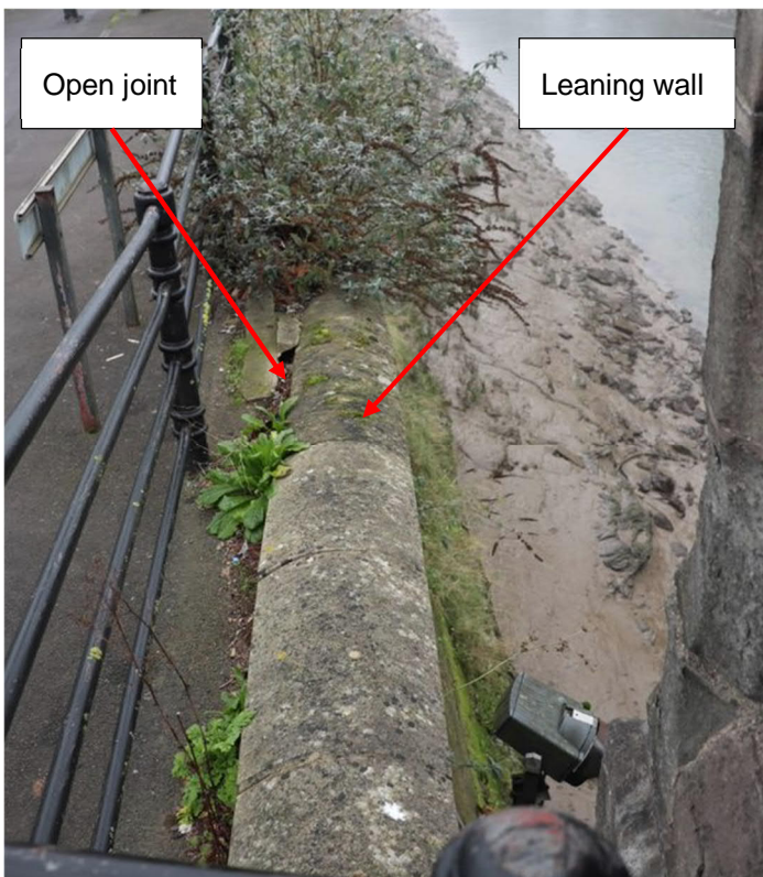
Figure 9.6: NCS21 Leaning wall
