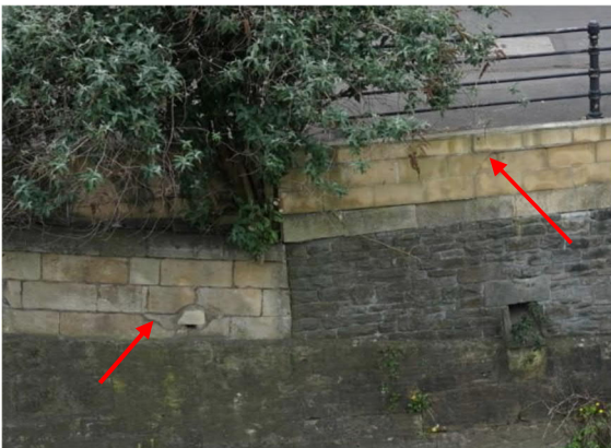
Figure 9.7: NCS21 & NCS23 Wall deformation 2019
