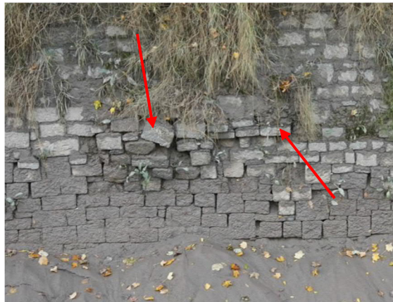
Figure 8.11: NCS18 Wall deformation 2022
