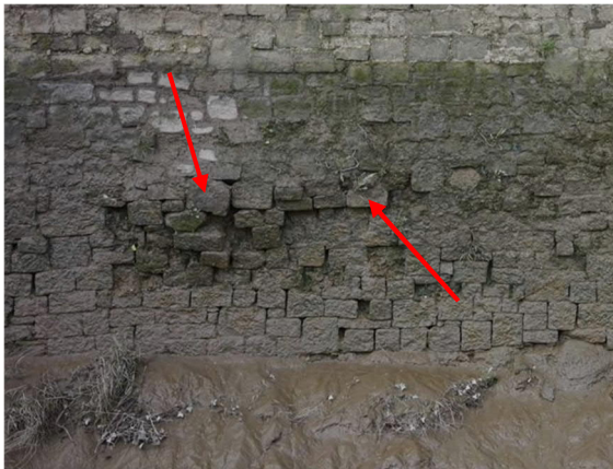
Figure 8.10: NCS18 Wall deformation 2019
