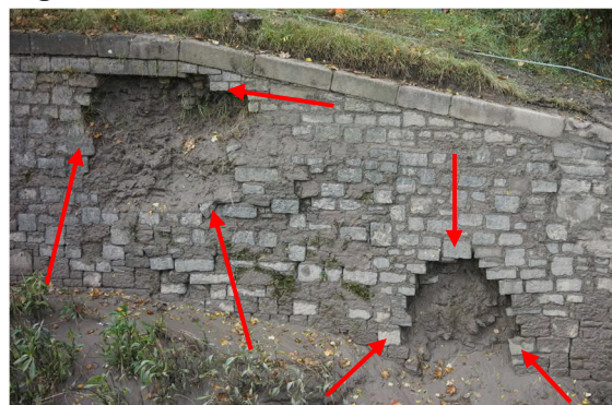
Figure 8.9: NCS18 Defect A and B 2022
