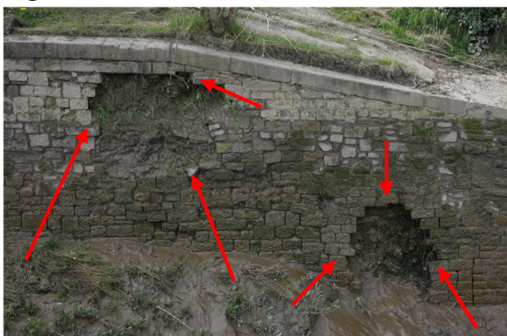
Figure 8.8: NCS18 Defect A and B 2019
