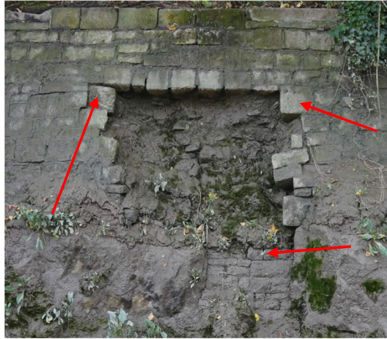
Figure 7.8: NCS13 Collapsed section 2022
