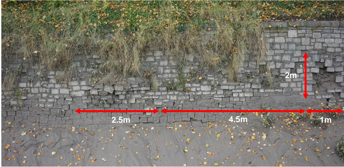
Figure 8.5: NCS18 Wall deformation and lost masonry (Slope wall)
