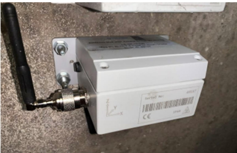
Figure 2.1: Wireless 3D tilt node fitted directly to concrete structure
