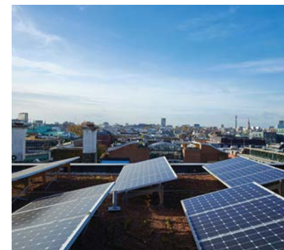
Integrated on-site energy production and biodiverse roofs
