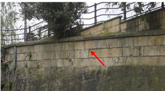
Figure 9.9: NCS21 & NCS23 Leaning wall 2019
