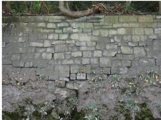
Figure 7.10: NCS13 Wall deformation 2022
