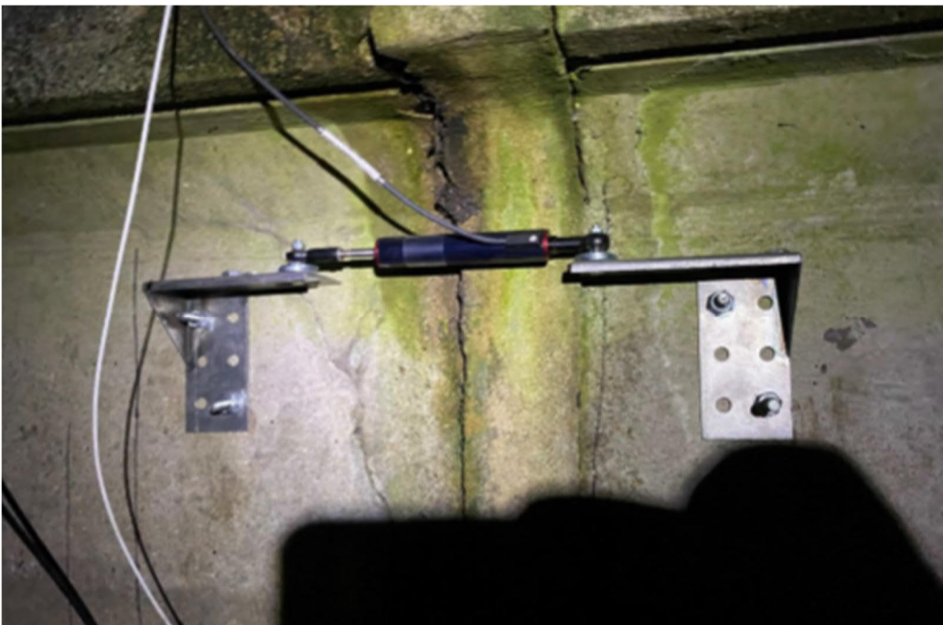
Figure 2.3: Typical linear displacement sensor across crack
