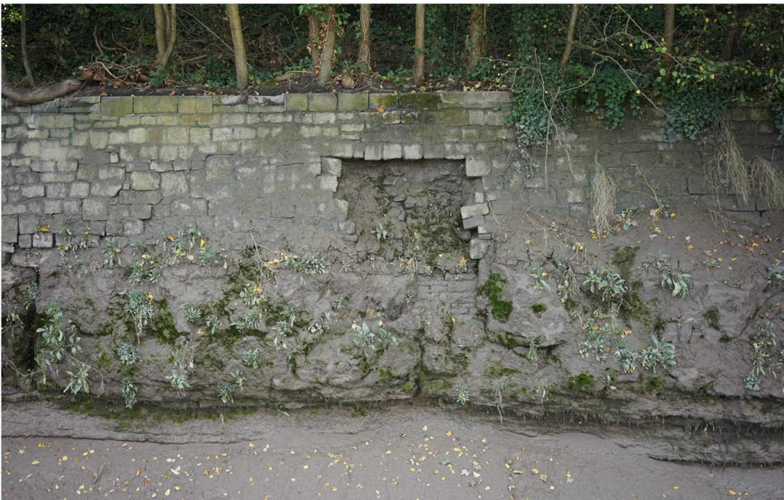
Figure 12.5: NCS13 Collapsed section
