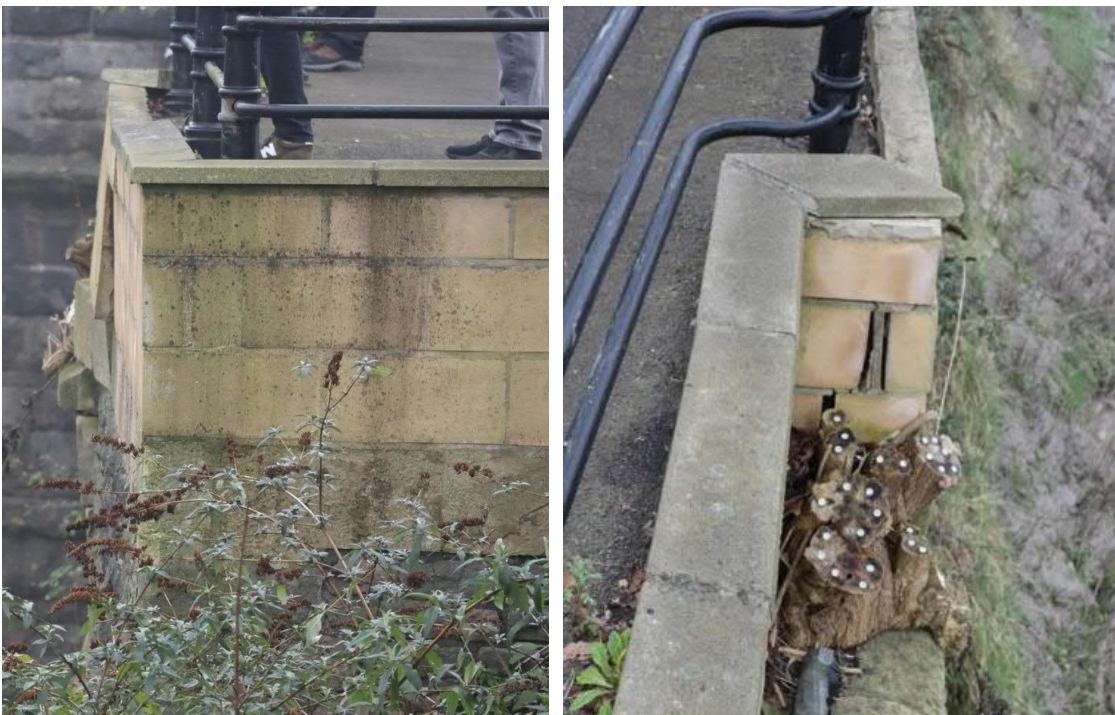
Figure 9.4: NCS21 & NCS23 Wall deformation
