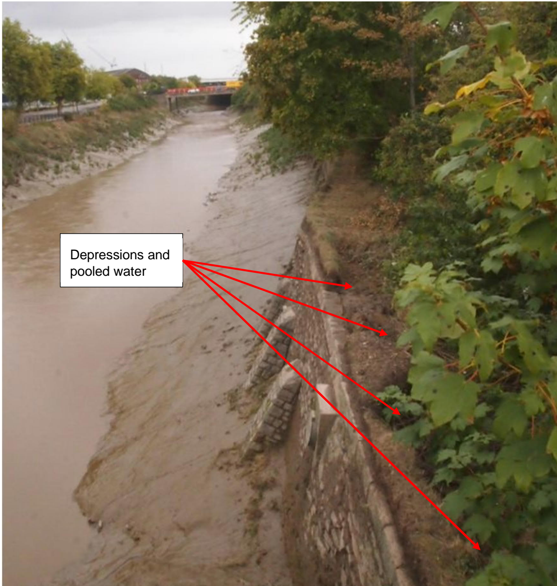
Figure 10.14: NCS28 Upstream depressions behind wall
