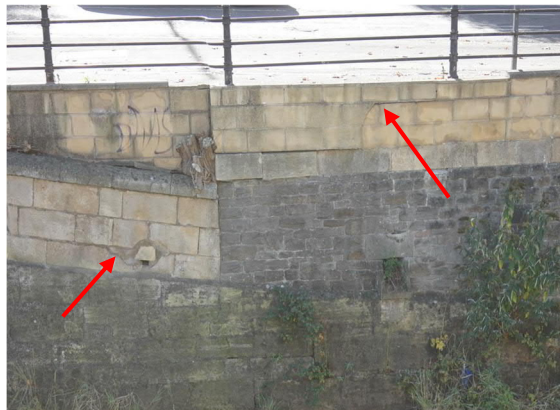
Figure 9.8: NCS21 & NCS23 Wall deformation 2022
