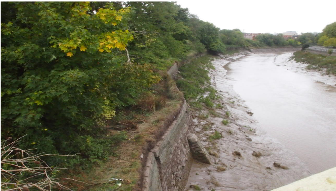
Figure 10.10: NCS28 Downstream area of deformation view from the bridge
