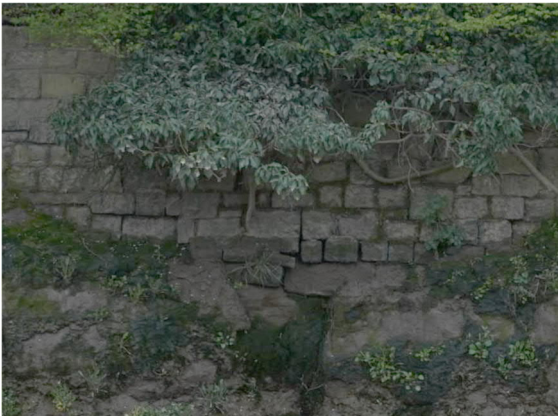
Figure 7.9: NCS13 Wall deformation 2019
